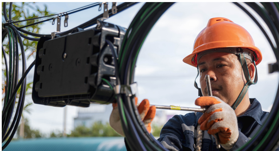
As a managed services partner, Spectrum Enterprise regularly services and updates the data aggregator's network to ensure it carries a steady and secure flow of information.
